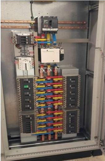
SMBD with Leakage Relay & Toroid
