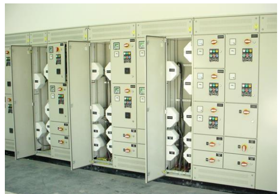
Motor Control Center Form-4 Type-6
