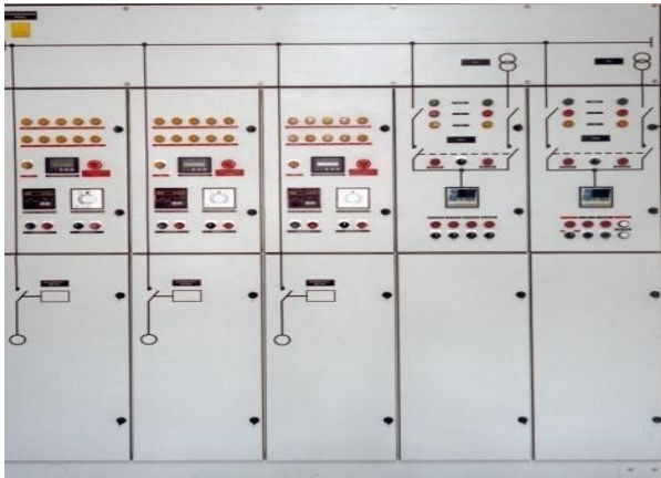
Synchronizing Panel 3x500KVA plus 2 ATS Form-3B
