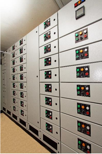
Motor Control Center
