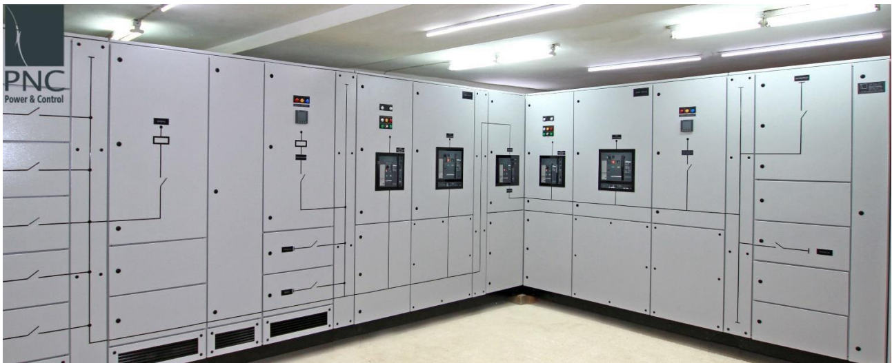
BUS-TIE 1600KVA With 2xATSS-MDB, Between EDL & Synchronizing, Form-3B
