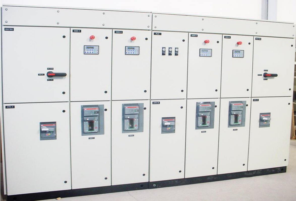
Synchronizing And Bus-Tie Panel Form-4 for shopping Center
