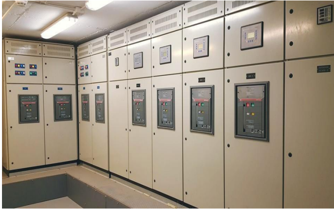
Synchronizing, ATS and MDB panels Form-4 for Hospital
