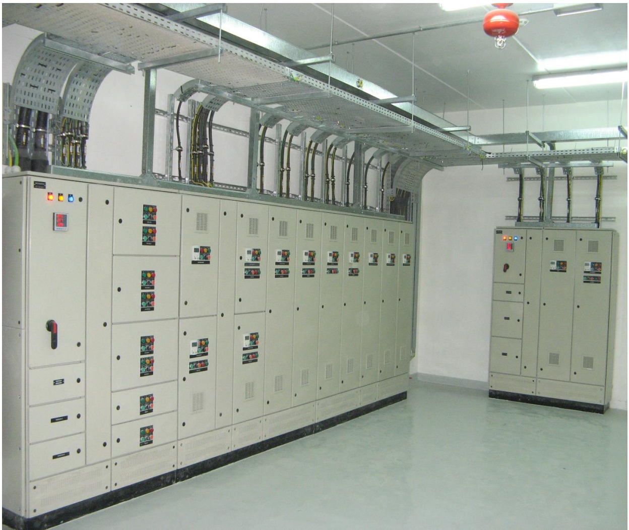
MDB and Capacitor Bank Form-4 for Shopping Center
