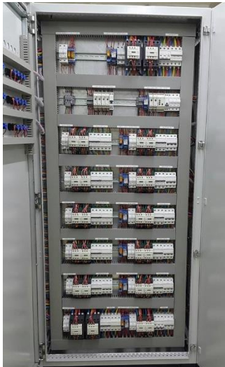
ATs Panel for residential Bldg.
