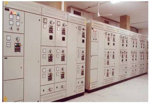
Motor Control Center Form-4 Type-6
